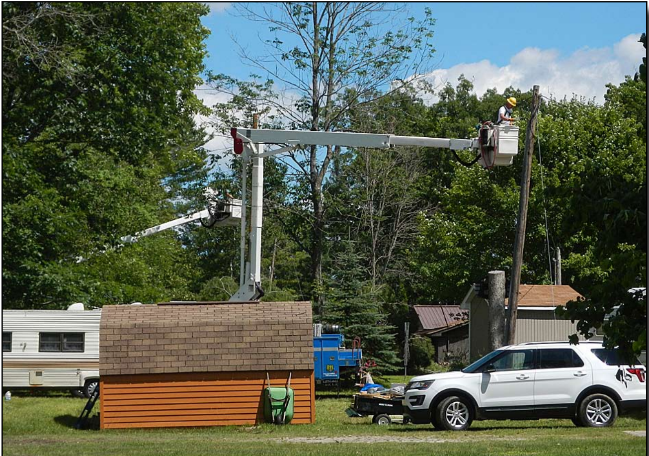
Consumers Energy crews repair power lines after strong winds buffeted the Hardwood Lake area Thursday, July 6th. Several trees came down and some homes received damage. Power was out for a couple days.
