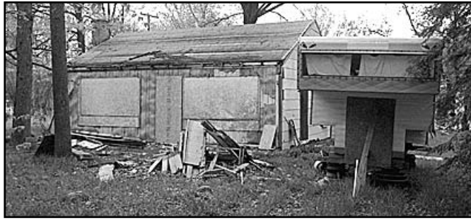
An empty lot exists (in foreground of bottom photo) where the dilapidated house on Hardwood Heights once stood (top photo).
